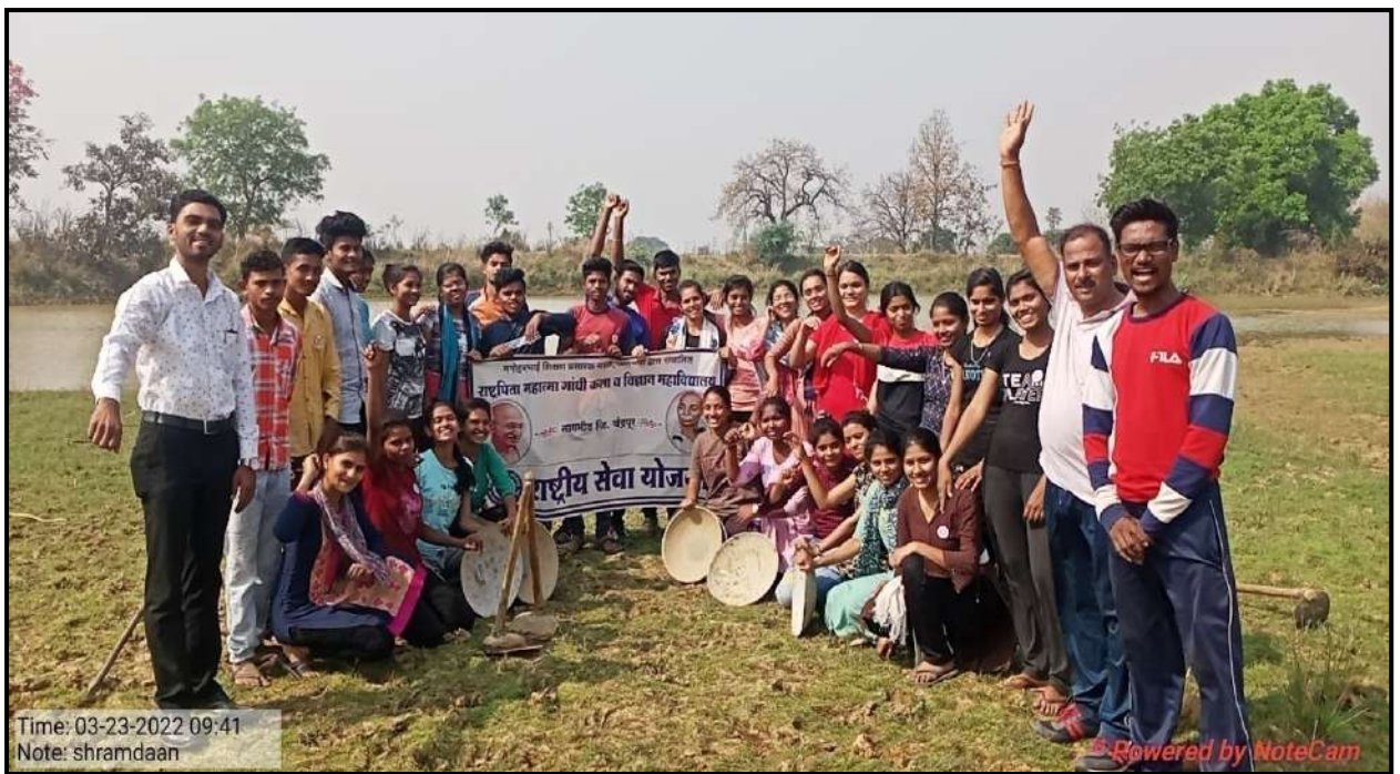
The NSS Volunteers Constructing a dam for the villagers on dated 23 March 2022
