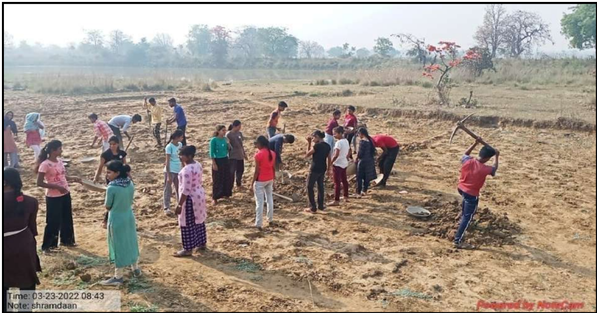
The NSS Volunteers Constructing a dam for the villagers on dated 23 March 2022
