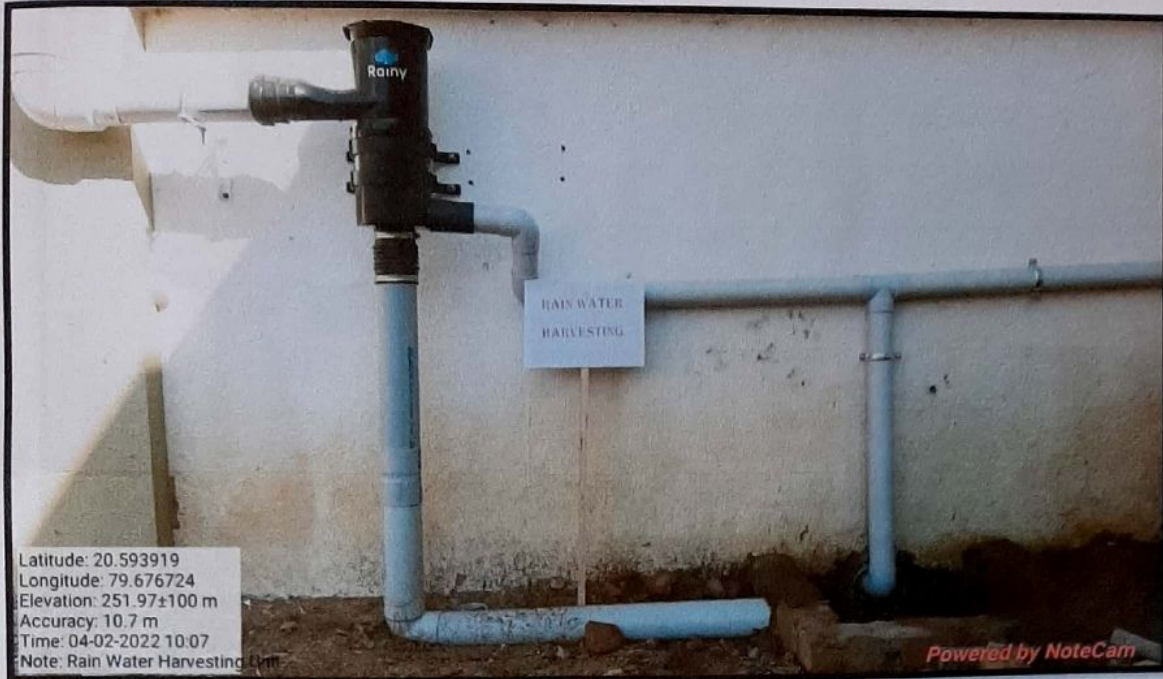
Rain water Harvesting Unit
