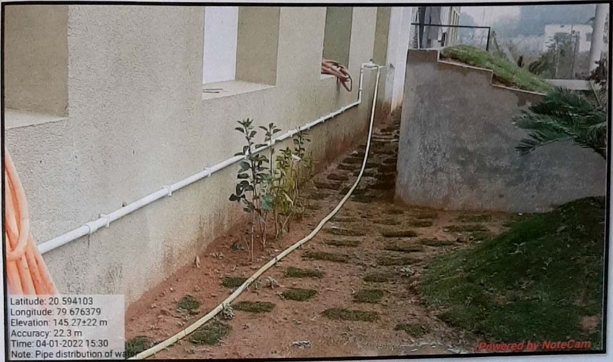
Water supply through pipes in Garden
